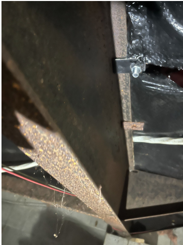
Steel bracket bolted directly to the home's steel frame.
