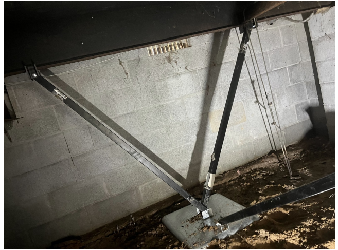
Steel 'V' brace anchored into the ground — keeps the home from shifting front-to-back.
